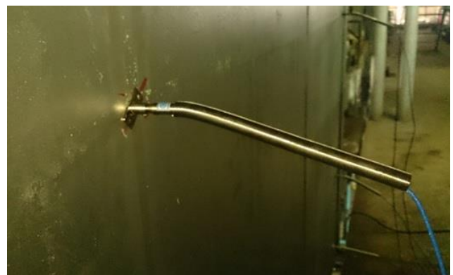
Fig. 10. The K-type thermocouple installation on the oven wall.
