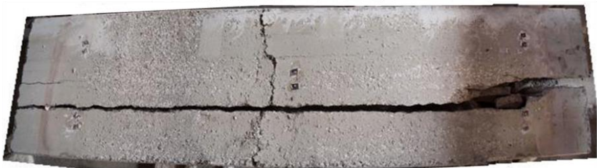
Fig. 18. HCL5 after fire test.
