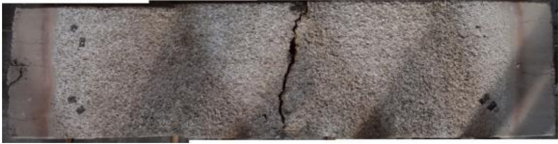
Fig. 14. HCL1 after fire test.
